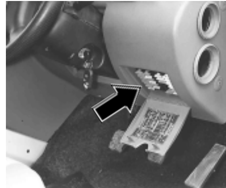
Fuse Box - Cabin
