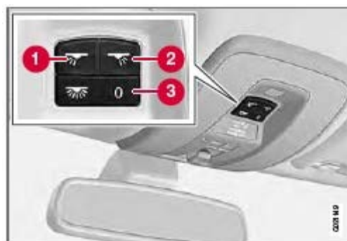
Light switches, front roof lighting
